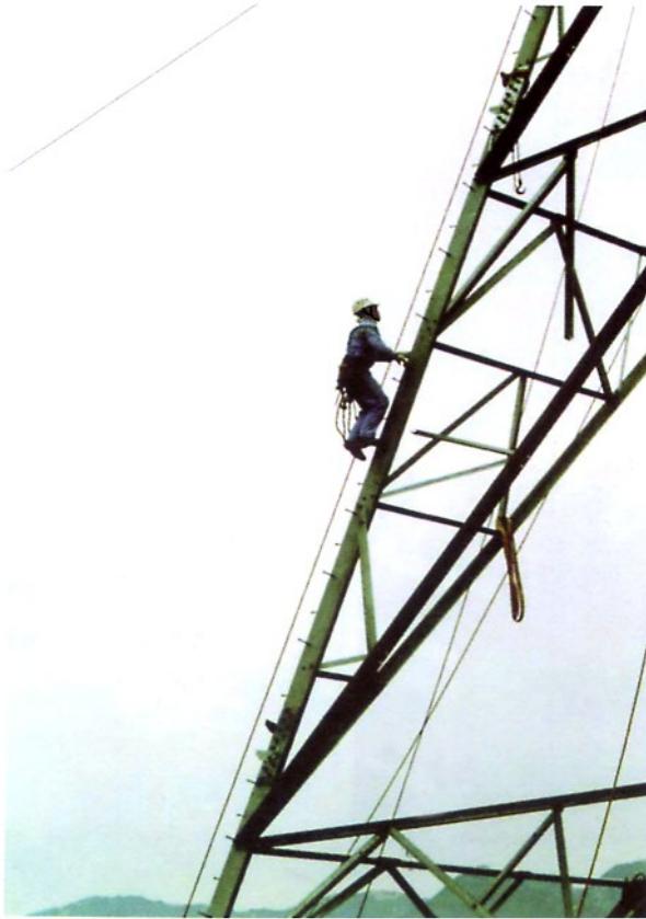
Photo 6 - electrical tower assembling work using guide rope, rope grab and rope adjuster
