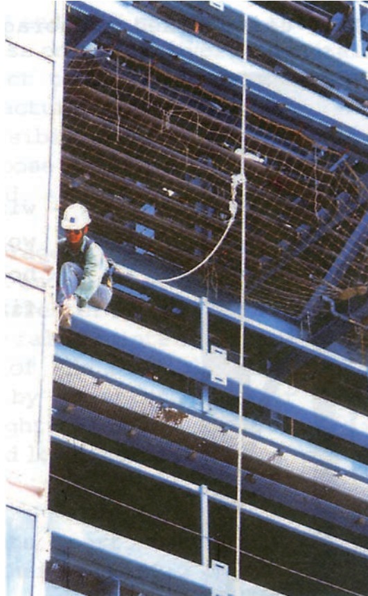
Photo 3 - external window panel installation work using rope chuck and vertical independent lifeline
