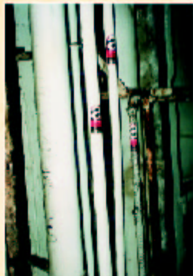
Boiler and pipe lagging
