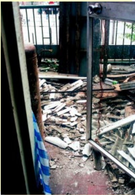
Asbestos containing materials should not be demolished without adequate worker protection.
