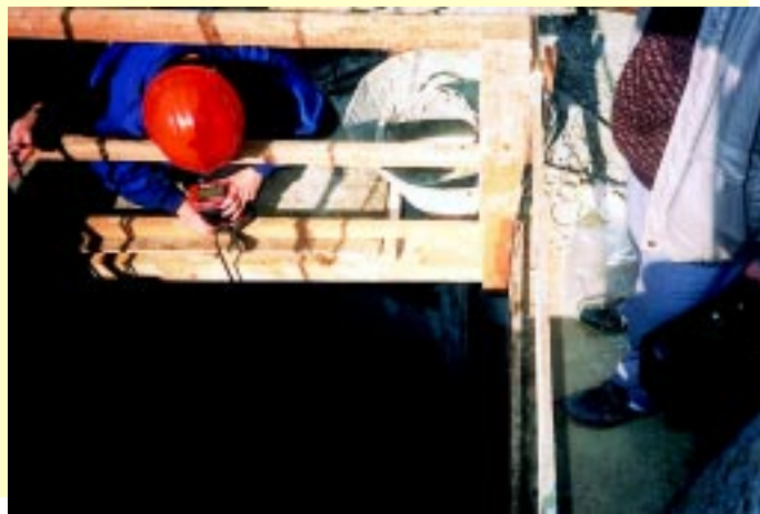
Monitor for hazardous contaminants before entering a confined space.
