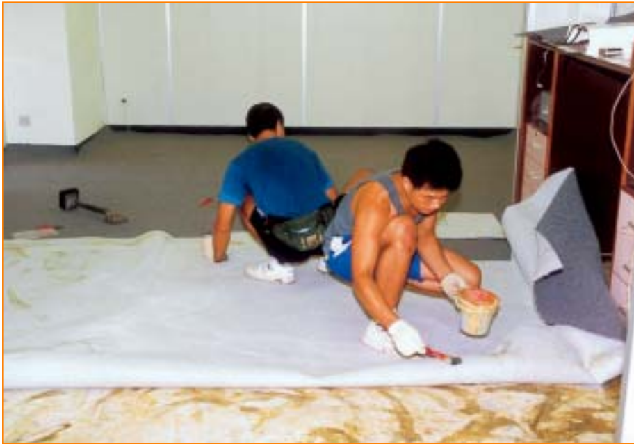
Carpet laying emits harmful organic solvent vapour into the air. The work area should be isolated from other office space.
