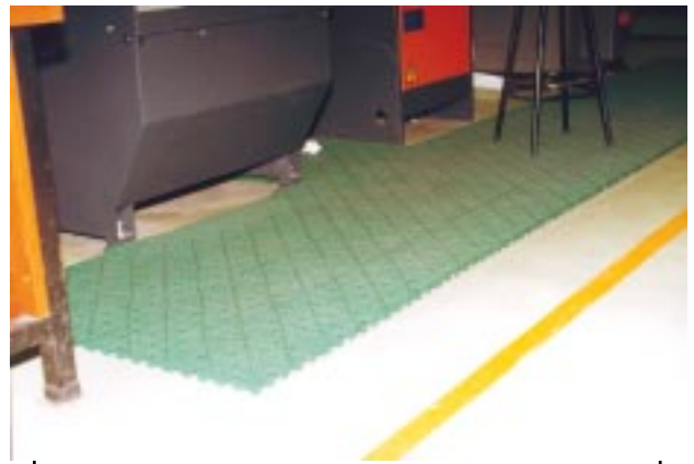
A raising platform should be provided where wetting of the floor is unavoidable, e.g. in an electroplating factory.
