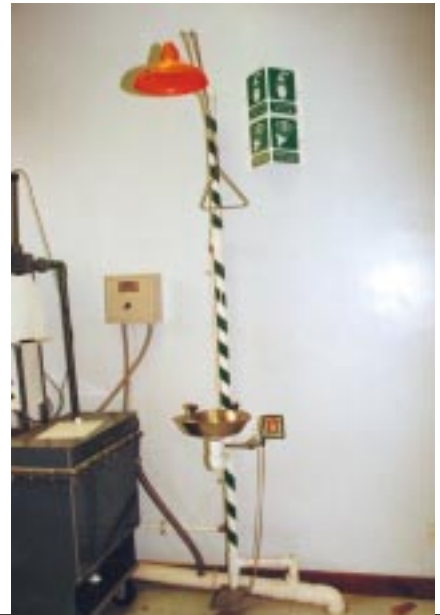
Emergency showers and eye washers should be provided in areas where accidental contact of the body with dangerous chemicals is possible.
