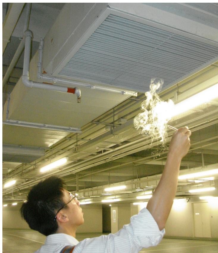
An occupational hygienist using a smoke tube to test the ventilation system at a car park
